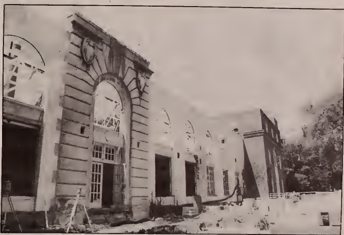
The landmark stone entrance on the West side of The Louis E. Reber Mechanical Engineering Building at University Park will soon disappear as part of a $13.4 million renovation. Construction crews have gutted the central portion of the building and will add a third floor dedicated almost exclusively to new, state-of-the-art undergraduate laboratories. The project adds approximately 10,000 square feet to the existing structure, which dates back to 1920 and was last remodeled in 1949.
